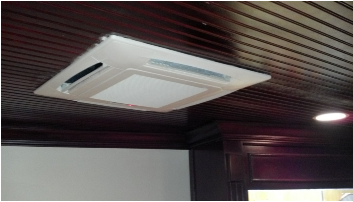
One of Six GPS-300 Units Mounted In Ceiling
